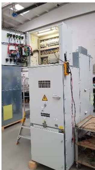
Fig. 2. 10 kV measurement cell.
